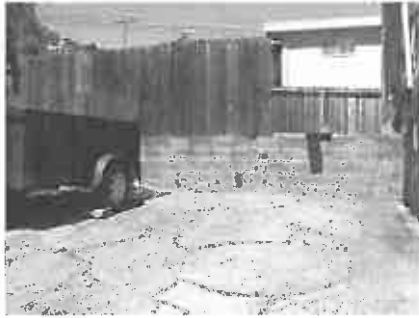
View of the existing CMU block wall as viewed looking up the driveway.
