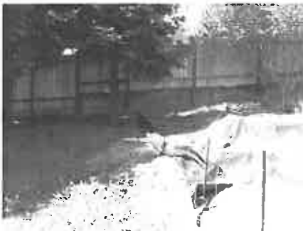
A large rectangular area of excavated soil is stockpiled under a tarp in the rear yard under the canopy dripline of at least one of the three trees in that corner. All of this material will need to be removed by hand using hand tools only, prior to erection of the root protection zone fencing perimeter.
