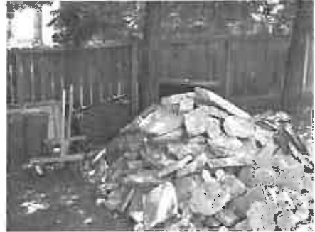
A full view of the concrete rubble currently stored under the canopy driplines of trees #1, 2, and #3. All of this material will need to be removed by hand only using no machinery.
