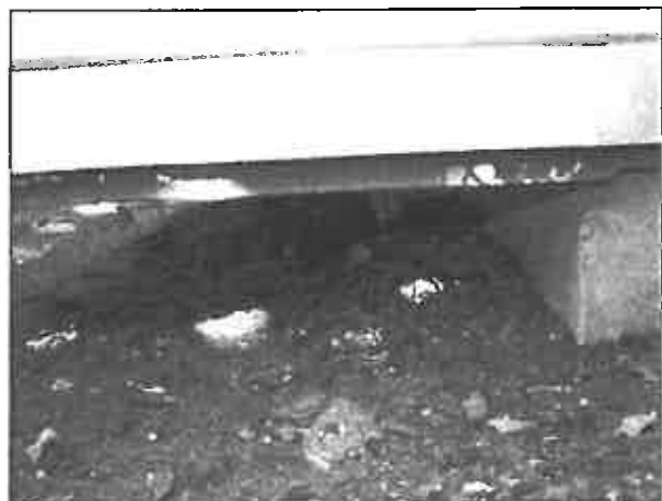
Right: Cantilever foundation in Palo Alto, set approximately 1 to 2 feet above grade.
